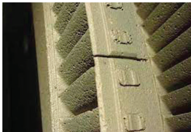
Fig. 1. Turbine blades damaged by erosion [7]
